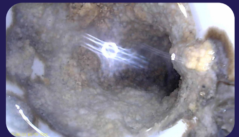
Urinal before, 3 rd floor in Caldecote building
